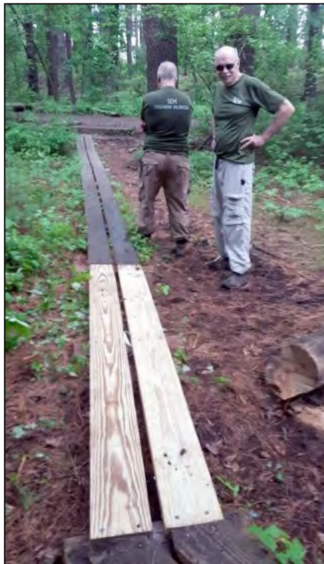
Pete Tierney inspects a section of new lumber replacing broken boards on the boardwalk.
