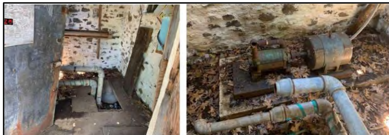
Interior, left, old pipes, pump, and motor, right.
