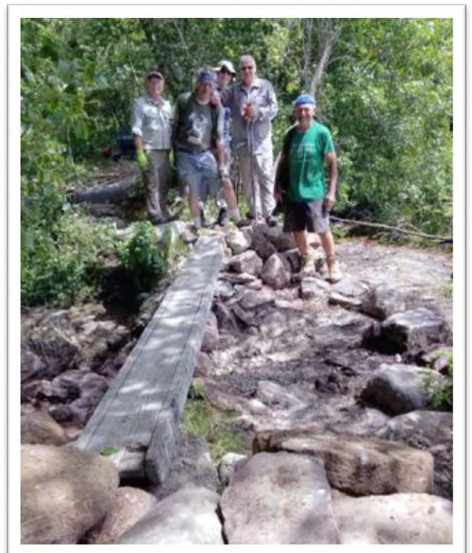
A hardy work crew constructs the fieldstone abutments at both ends of the planned new bridge. The old wooden single plank bridge in the photo will be replaced with a new wider bridge. Left to right: Skip Maysles, Bob Vogel, Pete Tierney, Paul Brookes, Charlie Farrell. Photo by Barry Young
