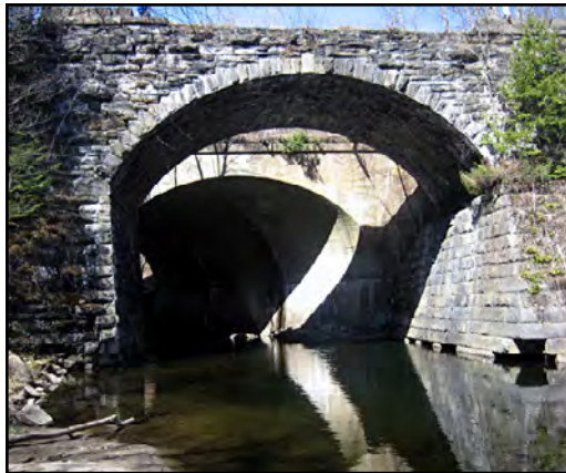
Keystone Arches Bridge with modern concrete version in background. Courtesy of Len Ulbricht
