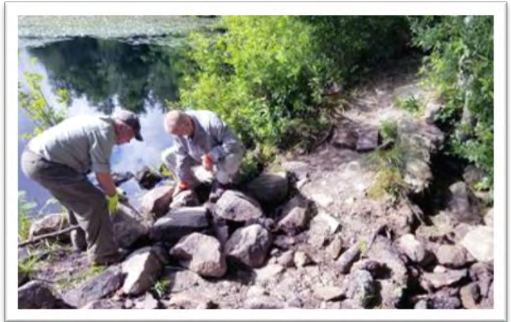
Skip Maysles, left, and Paul Brookes, right, move field stones to build the bridge abutments at both ends of the bridge span. Photo by Barry Young
